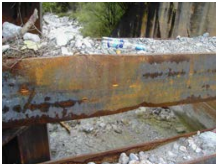
Deformation an Balken (SKL U) ©Suda
