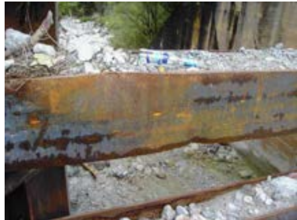
Deformation an Balken (SKL U) ©Suda
