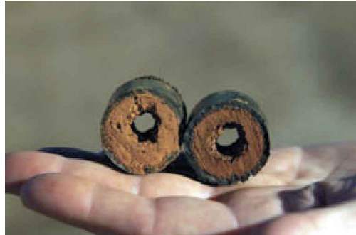
Figure 51. Drains subhorizontaux colmatés (document J.-C. Gress)
