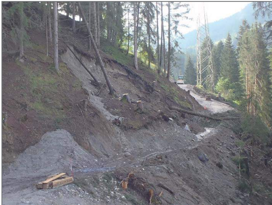
Rupture de talus amont (2014)
